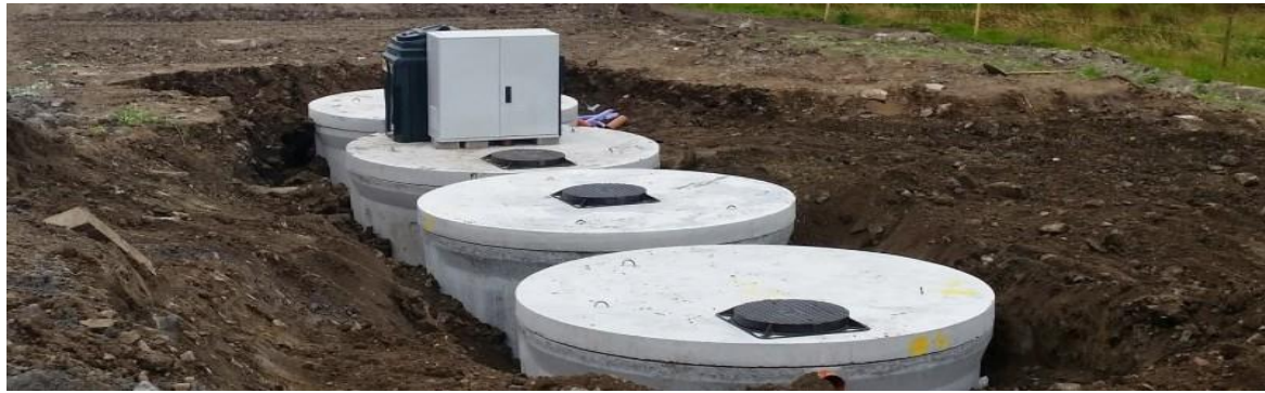
Figure 7.3: Septic Tank Riser
