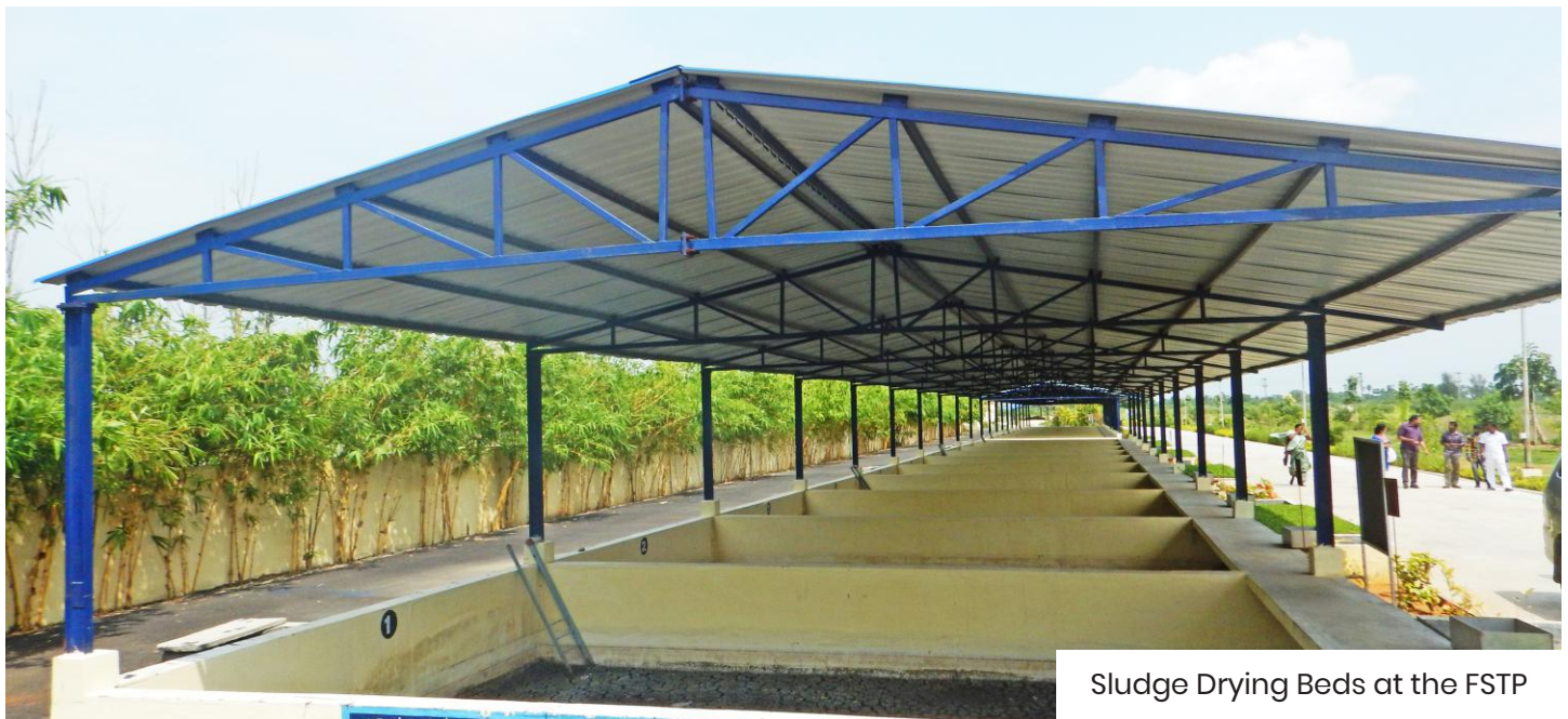
The raw sludge enters the Sludge Drying Bed
