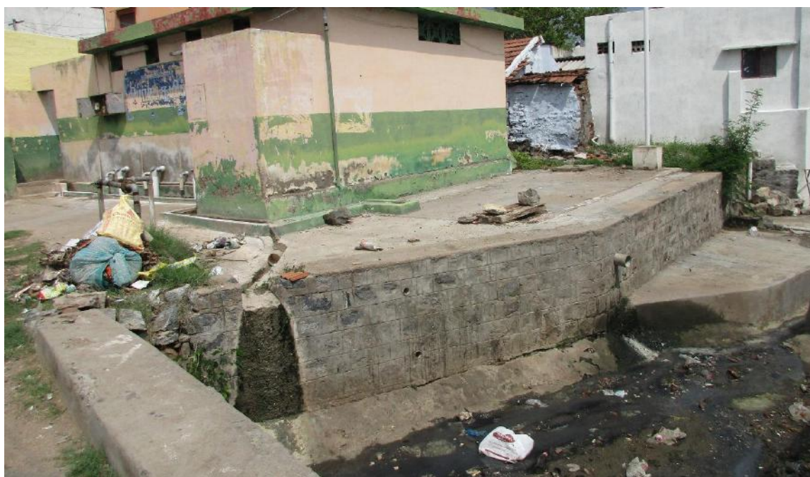
Figure 4.15: Household wastewater connected to open drains in Town Panchayat
