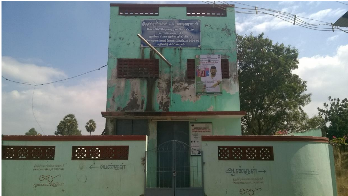
Figure 2.4: Toilet in Ward 41 K. Abhishekapuram Zone in Closed State
