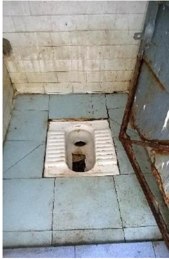
Figure 2.5: Pan Broken Rendering Toilet Seat Unusable
